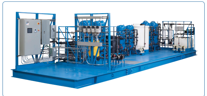
The above skid including pre-treatment, membrane de-gassing and distribution is deployed in a Steam Assisted Gravity Drainage (SAGD) facility in Western Canada.
